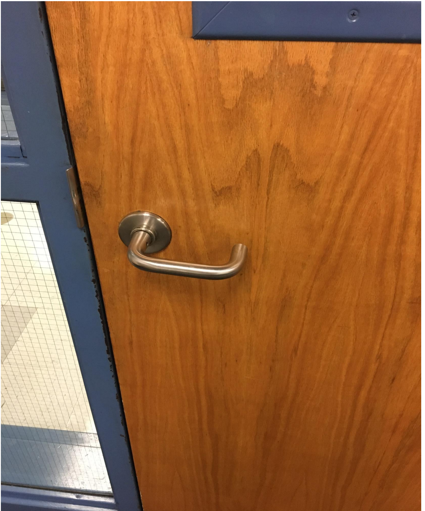
This is a picture of the interior of the door Mr. Cabrera allegedly locked in order to perpetrate the fictitious sexual assault on the student. (Note the absence of an interior deadbolt.)
